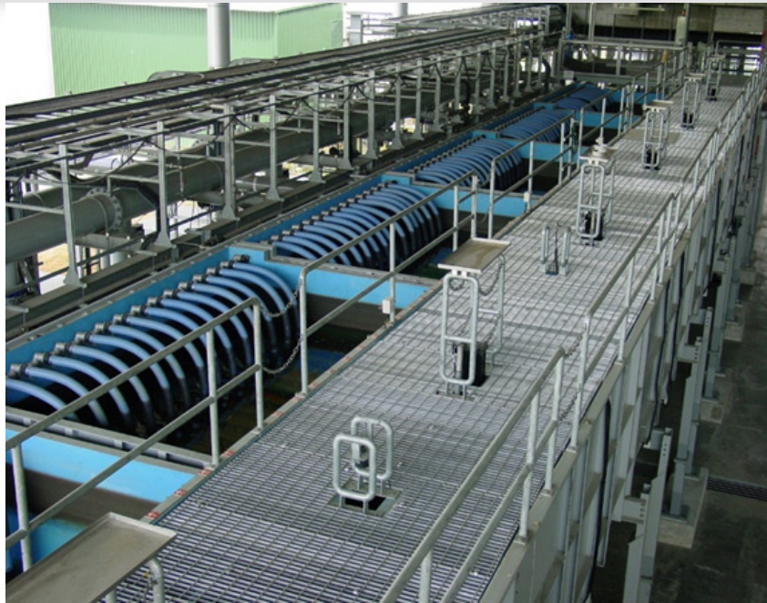
Ultra Filtration System at Kranji WRC
